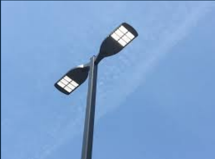
Shoe box type fixture in parking area
