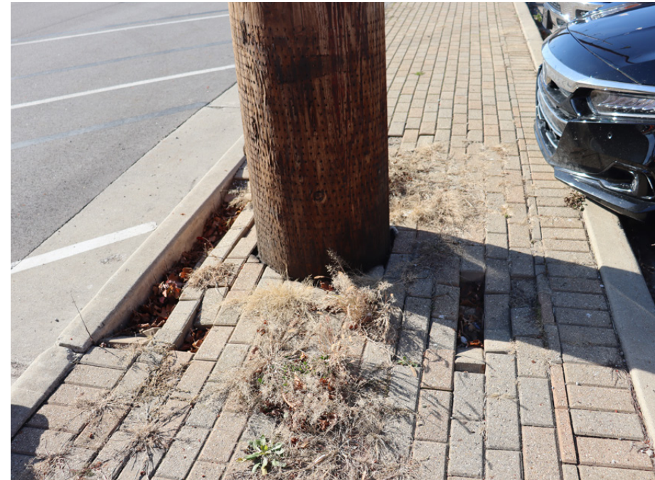
Existing Condition: Broken or missing pavers Opportunity: Remove and replace pavers where needed
