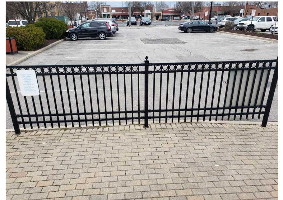
Existing Condition: Parking lot ornamental fence with sign Opportunity: Replace with new city standard for ornamental fence
