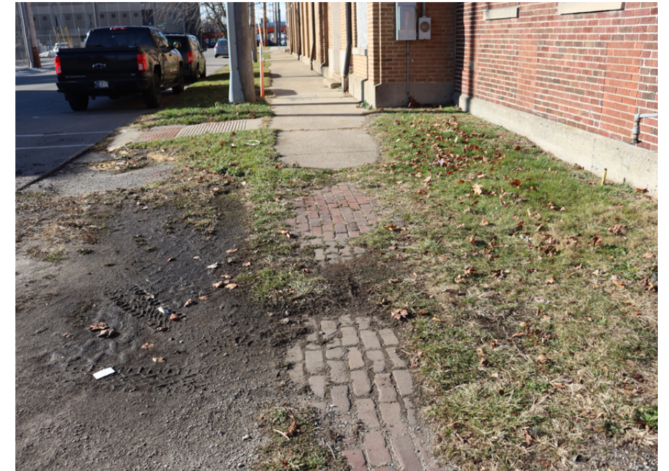
Existing Condition: Pavers are in poor condition with lots of settling Opportunity: Replace with concrete to follow the sidewalk aesthetic that is present on the site
