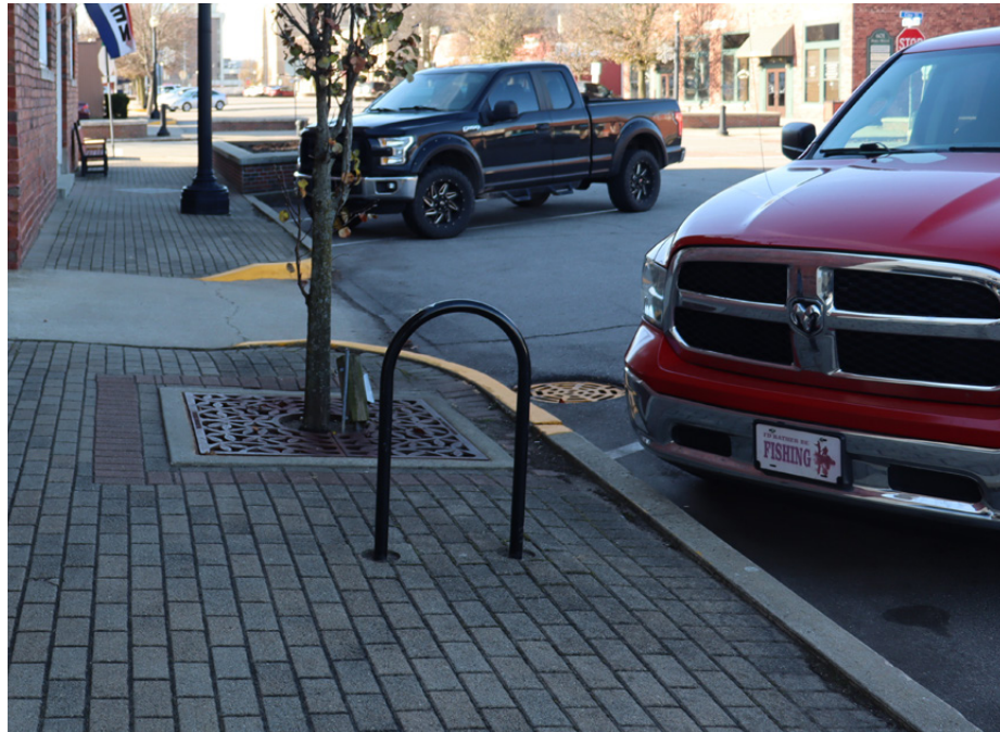
Existing Condition: Geometry, parking configuration, corner extensions adequate Opportunity: Configuration to remain, replace damaged curbs as required
