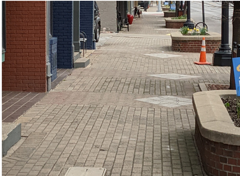
Existing Condition: Unit paving faded, some settling, most areas in good condition Opportunity: Replace areas with new paving
