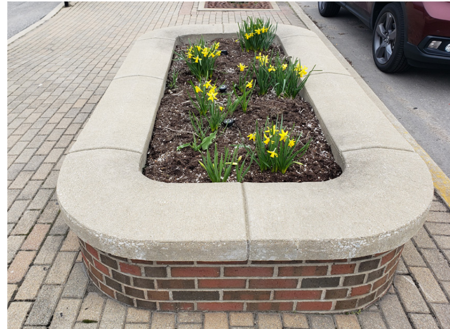
Existing Condition: Built in place masonry streetscape planter, shape and size vary Opportunity: Remove raised planters and replace with at grade planters with curbs
